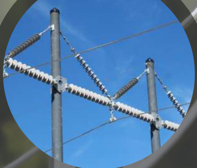
TOTALLY INSULATED FRAMING SYSTEM (TIF™) H-FRAME - TRANSMISSION 69kV - 230kV
